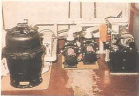
FILTRATION NEEDS ARE CRITICAL WHEN DEALING WITH POOLS FOR ANIMALS. SHOWN HERE IS THE PUMP AND FILTER SYSTEM USED FOR THE FERNO K-9 UNDERWATER TREADMILL. PHOTO COURTESY OF FERNO (WILMINGTON, OHIO).
